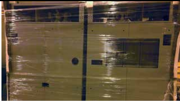
2 – Unused – Eaton AMPGARD SC9000 variable frequency drives Closes: 6/1 Contact: Troy Kidwell +1.512.784.1747
