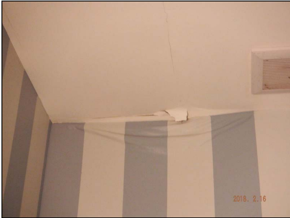
Photograph 27: Water damage observed in the main floor bathroom.
