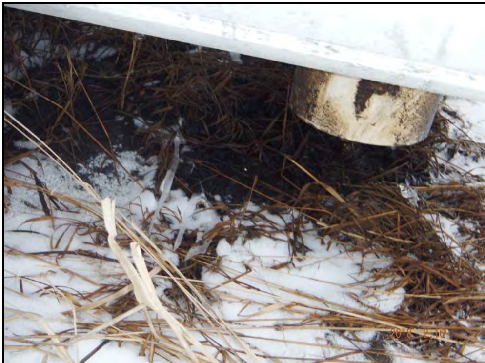
Photograph 24: Staining observed beneath the UN#1863 tank.
