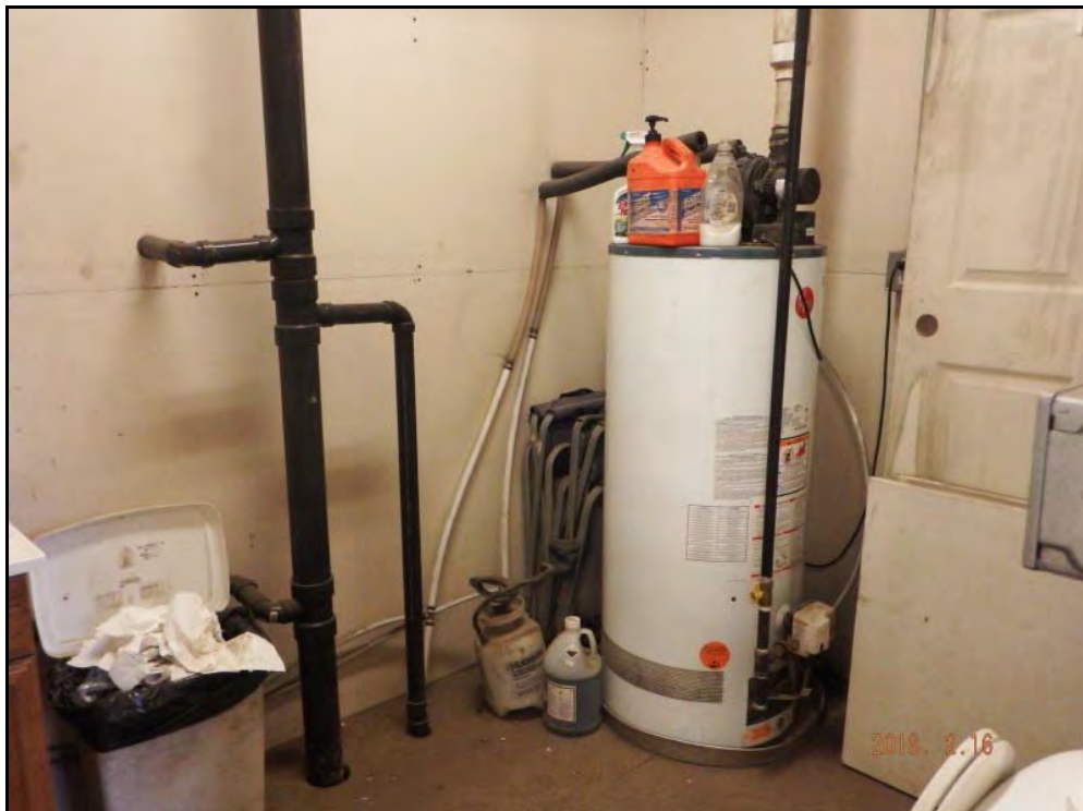
Photograph 30: Hot water tank and cleaning products observed on the loft.
